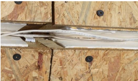
Figure G- 1 Romex wiring installation between roof panels in roof ridge prior to foam and ridge cap piece installation
